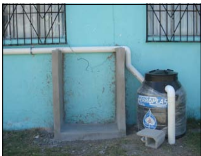
Scenes from Agustin Gonzalez. Gutters and water filtration are essential components of the rainwater catchment system.
