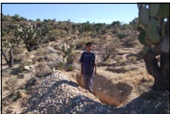
An erosion control and water infiltration structure is constructed in Ejido la Mesa, San Miguel de Allende.
